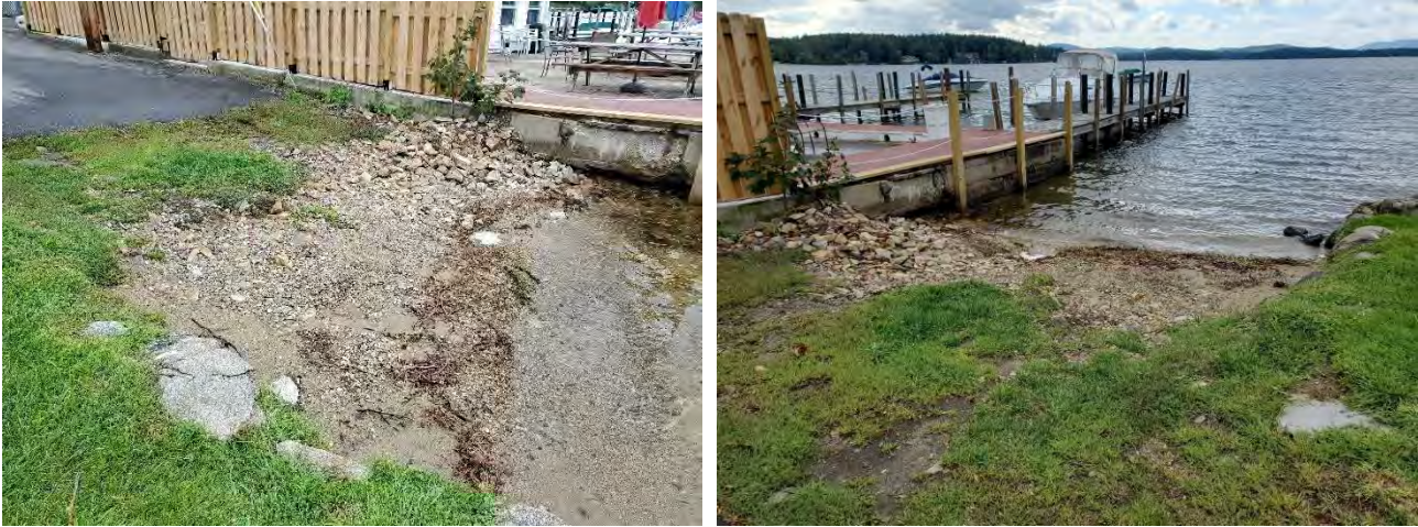
(Left) Erosion and bare soil at the water access point at the end of Lake St. (Right) Formerly grassy area is used as a boat launch.
