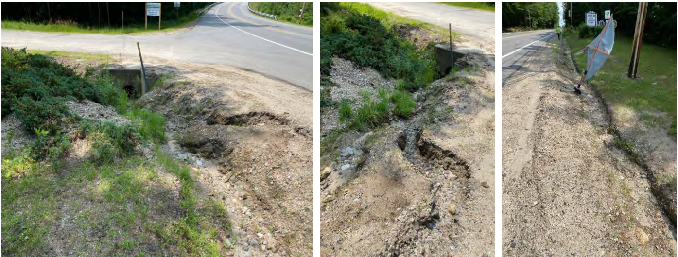
Examples of road shoulder erosion near Winnepesaukee Drive, July 2023. Photo Credit: FBE.
