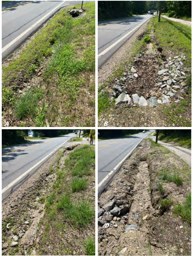
A, B, C, and D: Stormwater has eroded an existing road ditch, exposing bare soil and the tops of metal culverts. Sediment from the erosion ultimately accumulates in the catch basin near the bottom of the hill or continues moving downgradient.
