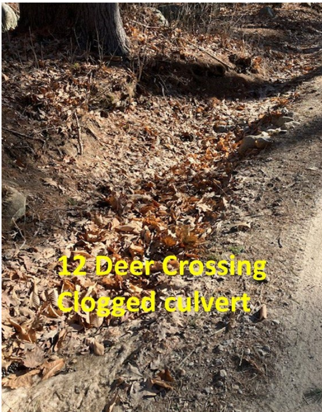
Caption: Clogged culvert at 12 Deer Crossing Rd.
