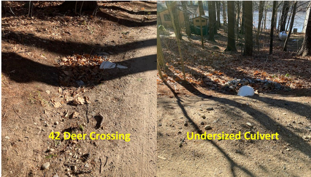
Undersized culvert at 42 Deer Crossing Road, Moultonborough
